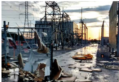
Merivale Transmission Station near Ottawa after a tornado destroyed the facility on September 21, 2018.
